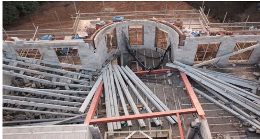
The scene after the collapse
